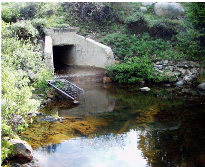
Below the dam, only leakage from the dam is allowed to flow back into the stream.
